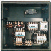
Interior View of MU-G20W FASD
