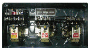
Interior View of MK1 SASD
