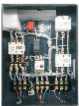
Interior View of MU-G30W FASD
