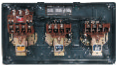
Interior View of MK2 SASD
